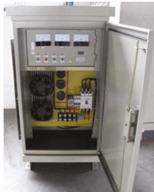
Fig. 7 Control cabinet of the submersible reciprocating pumping system
