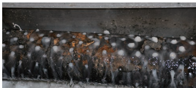
Fig. 11 Photograph of screen No. 5 flow after cleanup with mud acid
